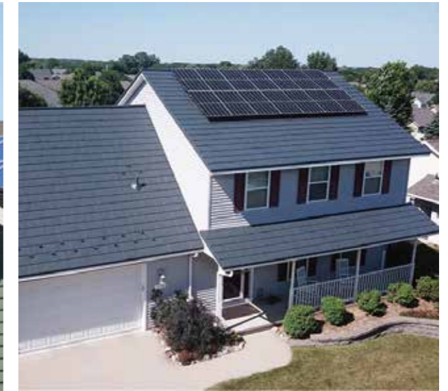
Residential Project in Philippines 3kW
