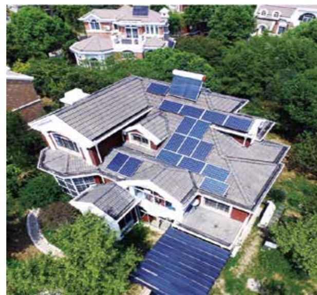
Residential Project in Philippines 3kW
