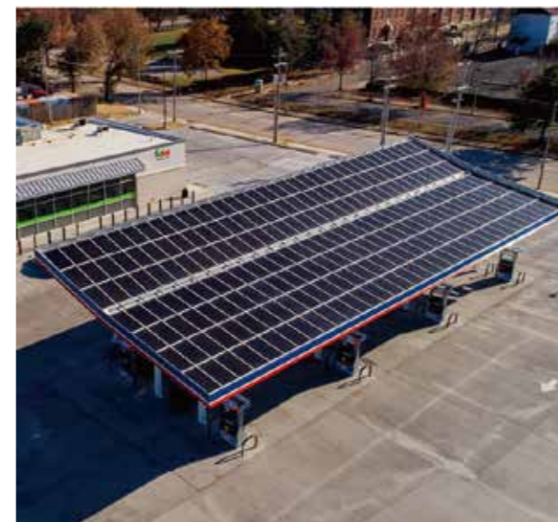
Gas Station Project in Brazil 26kW
