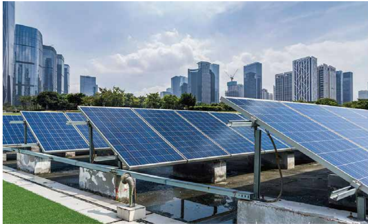
Residential Project in Sweden 10kW
