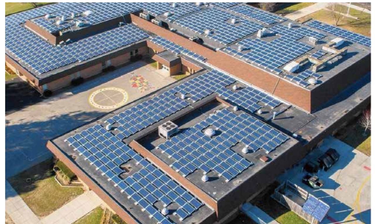
Industrial Project in South Africa 158kW
