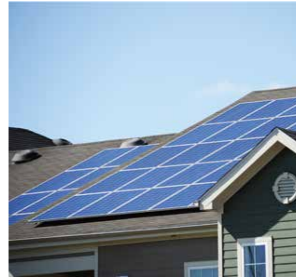
Residential Project in Indonesia 6kW
