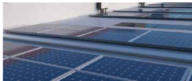
Residential Project in Poland 3kW
